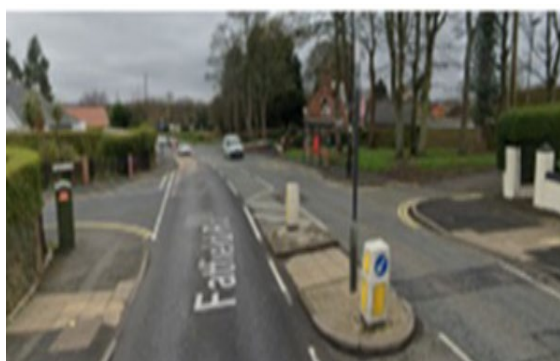
Pedestrian crossing facilities on Biddick lane and Fatfield Rd do not meet current guidance
