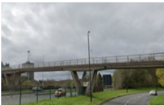
Access to Galleries via overbridge (~3m wide). At grade option likely not feasible due to A1231 crossing requirement.
