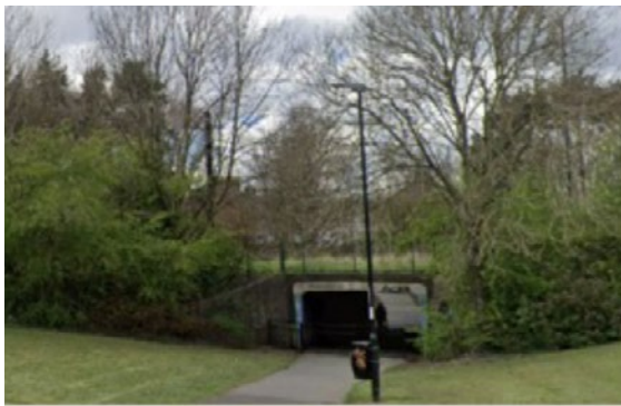
A195 underpass can feel secluded. Poor lighting / CCTV. Guardrail chicane causes obstruction to cyclists.
